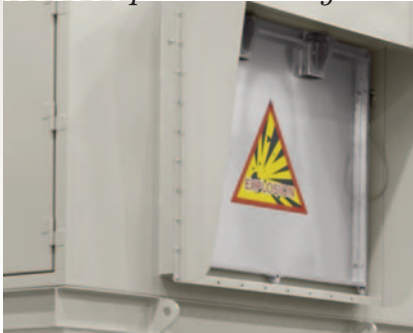
Explosion venting doors
